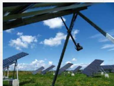
Former landfill site with 54 DEGERtrackers, Germany
